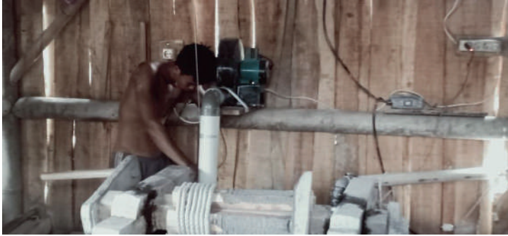
Photo 2.12 Ventilation System with Blower from Above
