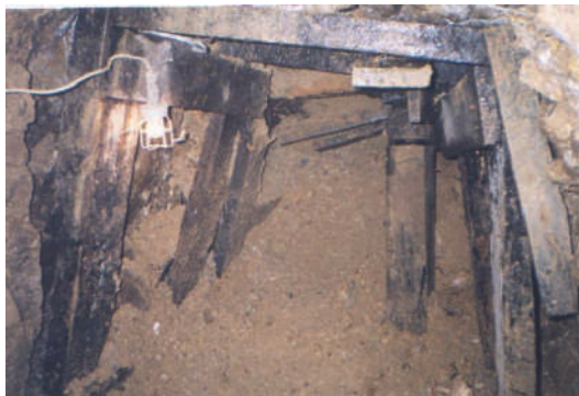
Photo 4.6 Collapse in Tunnel That Must Be Handled using Boring
