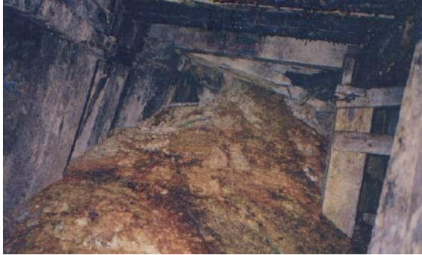
Photo 2.4 Collapse in a Tunnel
