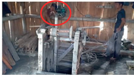
Photo 4.14 Simple Communication Tool using Ventilation Tube
